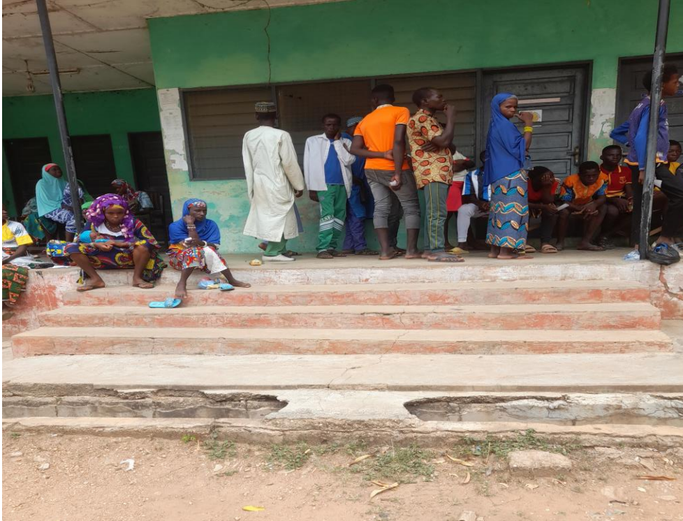
Photo Above: One of the registration centres in the Oti region with open gutters and steps at the entrance which makes it physically inaccessible.
